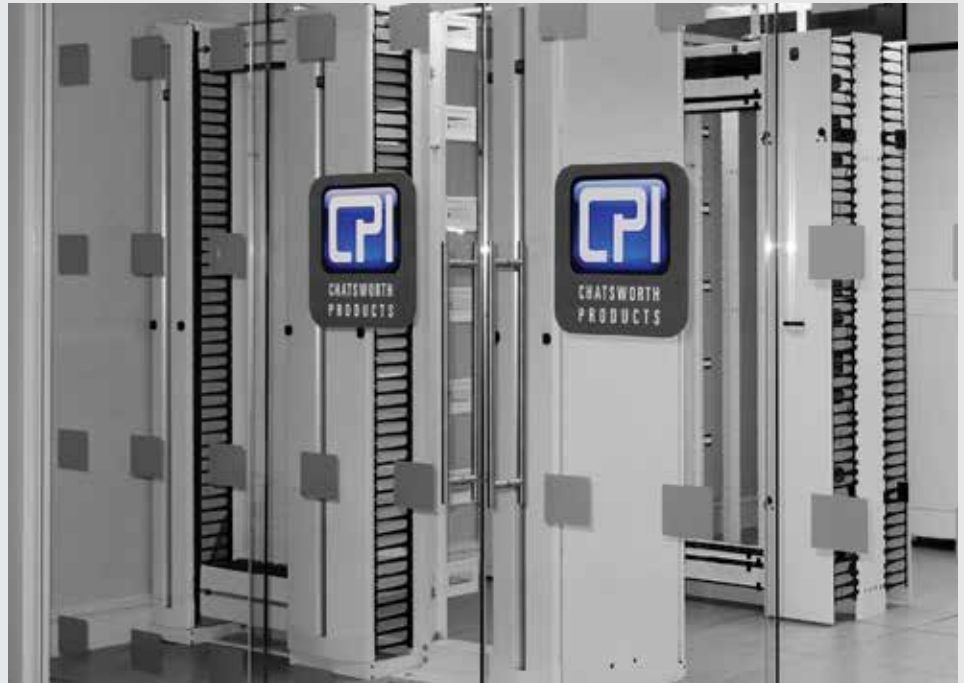
Data centre – unprecedented demand on IT systems in data centers is seeing network capacity go to 100 GB (Image: CPI)
