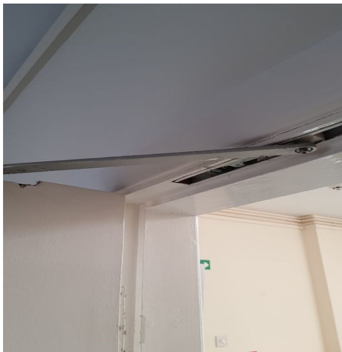
No.2 The hold open device fitted to the kitchen door should be removed and a self-closing device should be fitted.
