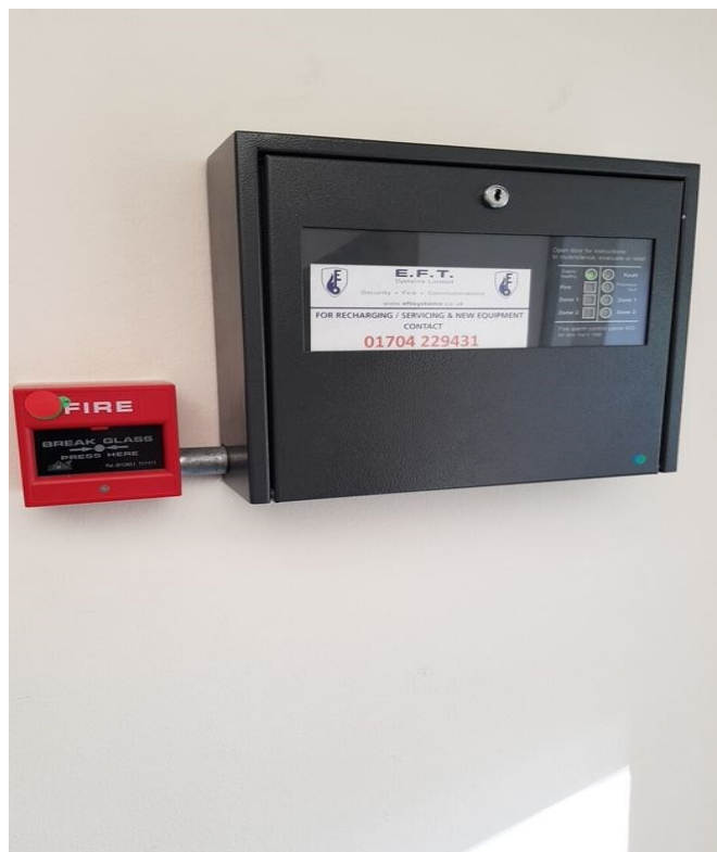
No.4 Display a fire alarm zone plan.
