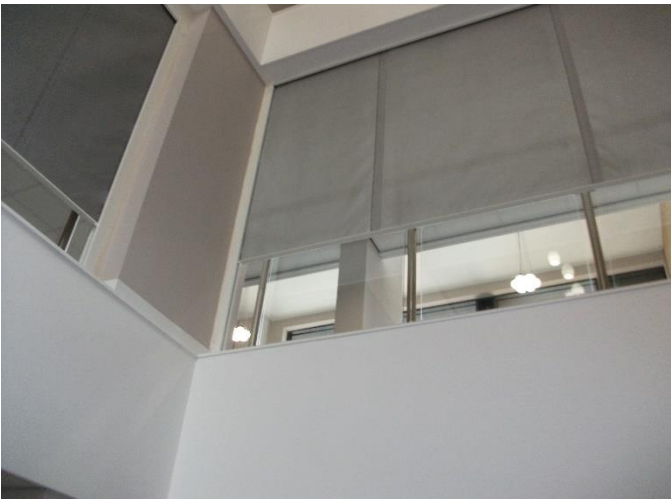
Fire curtains in atrium
