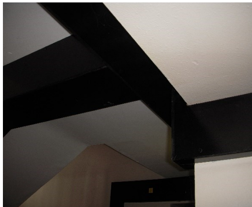
Electrical cabling in common areas in timber trunking
