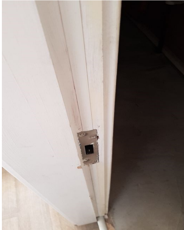
No.1 Replace the intumescent seals with intumescent smoke seals (electrical distribution room).
