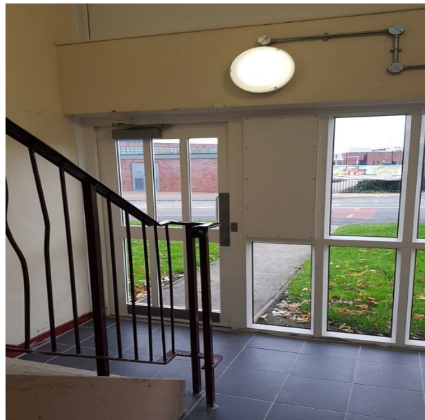
No.3 Display a Halton House specific fire action notice.
