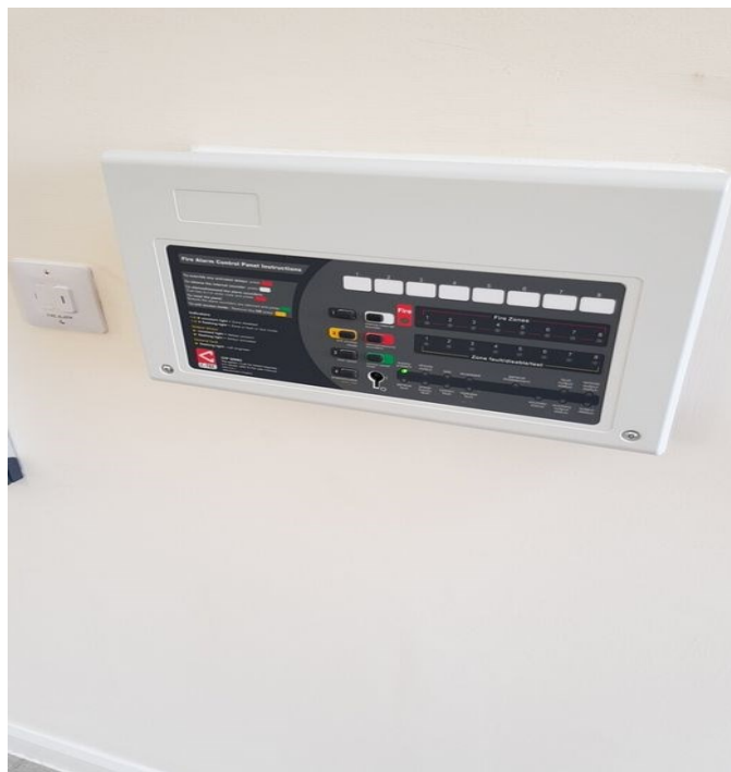
No.1 Display a fire alarm zone plan.
