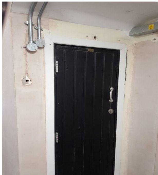
No.4 Repair the holes with materials that have a minimum of 30 minutes fire resistance.
