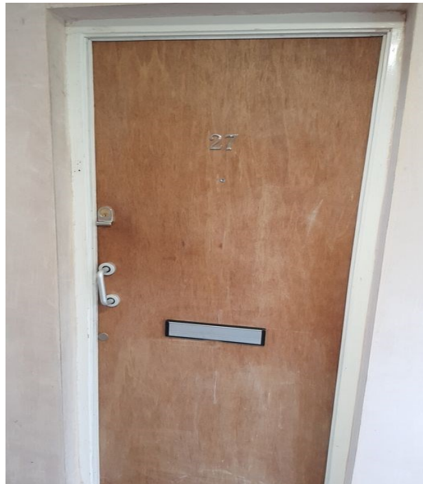
No.4 Replace the self-closing device.
