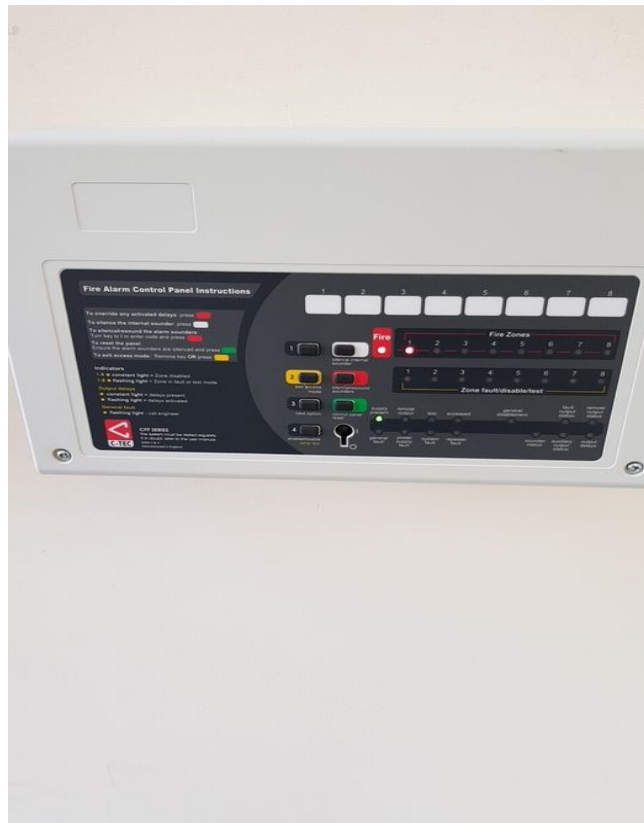
No.3 Reset the fire alarm panel.
