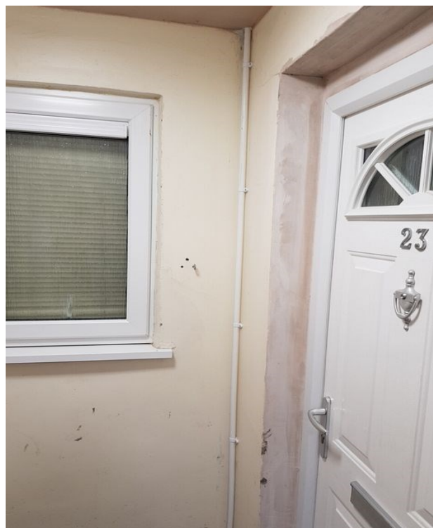
No.4 Investigate the fire resistance of the windows between flat 23 and the common area.
