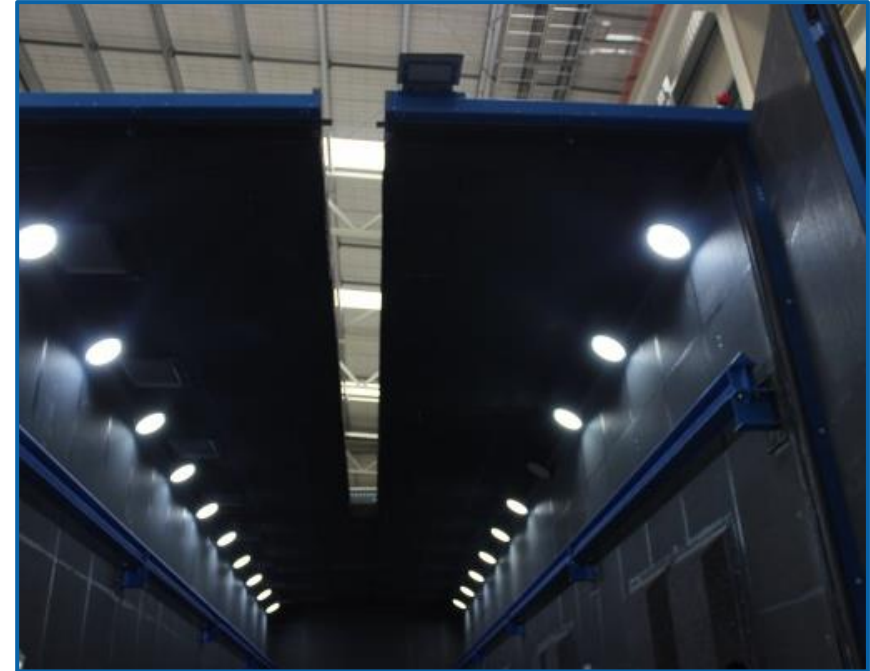
Roof slot 11 x 0.5 m, with driven roof flap, makes it possible to use a bridge crane.
