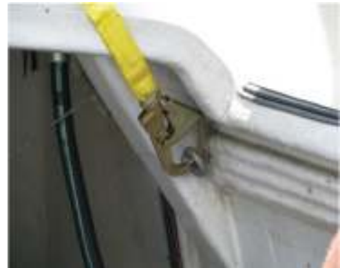
A single point anchor used while providing maintenance on a wind turbine.
