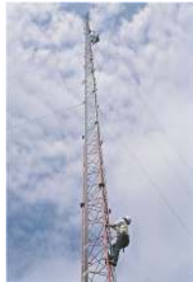
A worker using a vertical lifeline and ladder system while providing maintenance on a power transmission tower.
