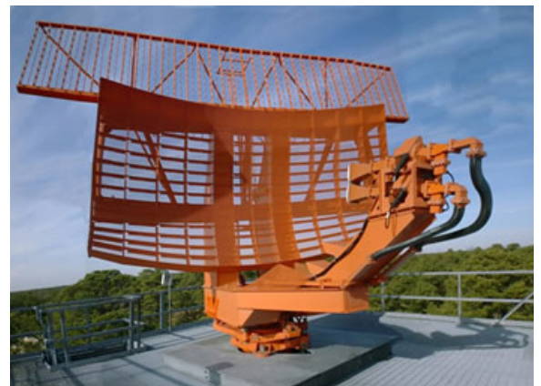
Figure 4: PQube is used to monitor remote ATC RADAR facilities
