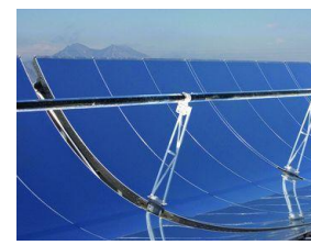
curved solar panels
