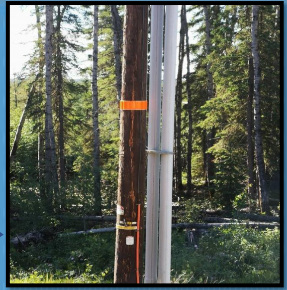
Close up of cracks
