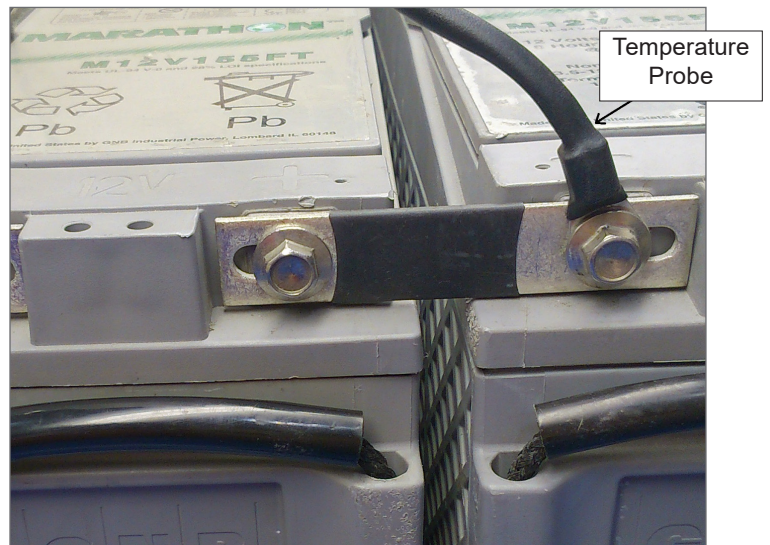
Figure 27 — Battery Temperature Probes—Battery Bay
