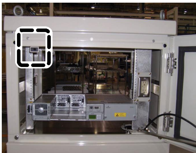
Figure 8: Door Intrusion Switch (typical view)
