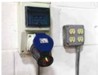
GREEN & RED lamps light: one phase is missing
