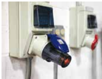
RED lamp lights: phase sequence is wrong
