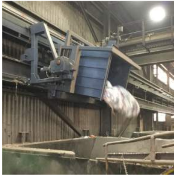
Figure 9 - WFS Dumping mechanism feeding MWC feed chute
