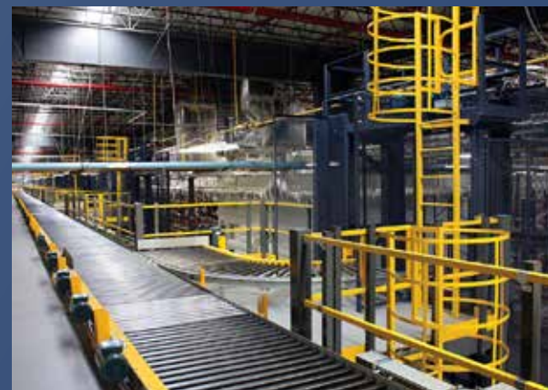
Home Appliance Lifts – M Series Mechanical VRC Ten lifts installed as a mezzanine application, including a conveyerized system. 1,200 lbs. lifting capacity; 200' per minute travel speed.
