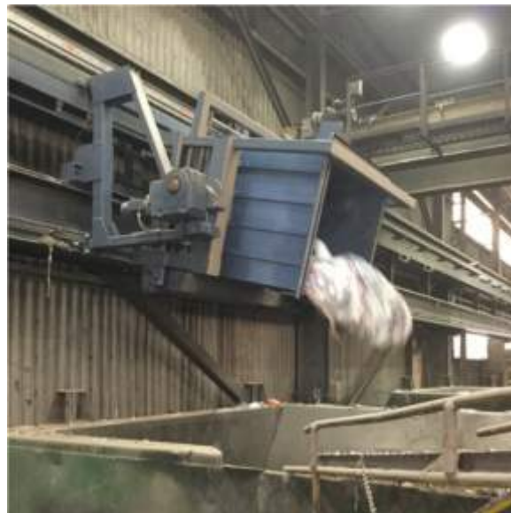
Figure 5.3.5 WFS Dumping mechanism feeding MWC feed chute
