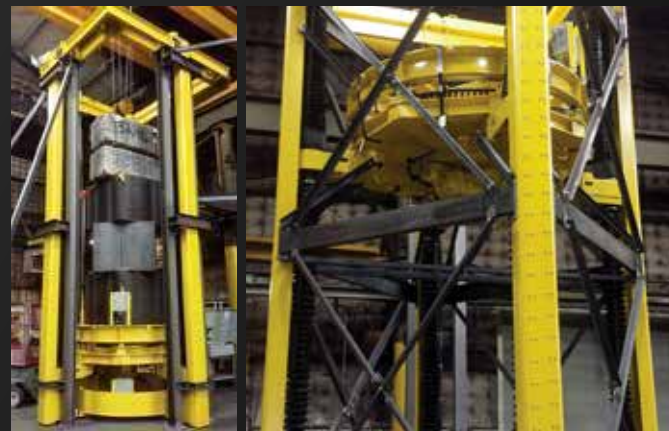
University Research – High-Capacity Lift – Custom 4-Post VRC This precise vertical and circular motion lift is installed in a scientific accelerator facility for nuclear science. 26,000 lbs. lifting capacity; 19' lift travel; 5' per minute travel speed.
