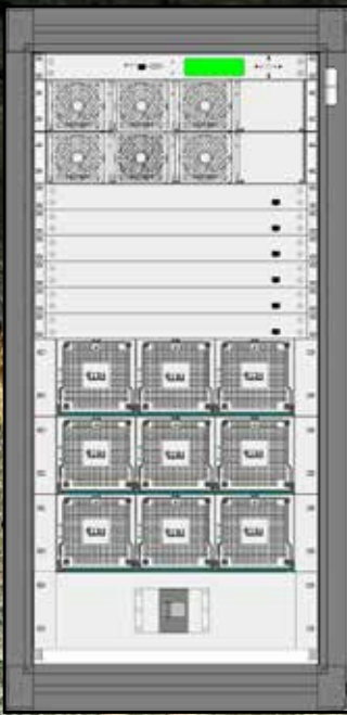
Example of 10kW UPS System with Lithium Ion Battery Backup
