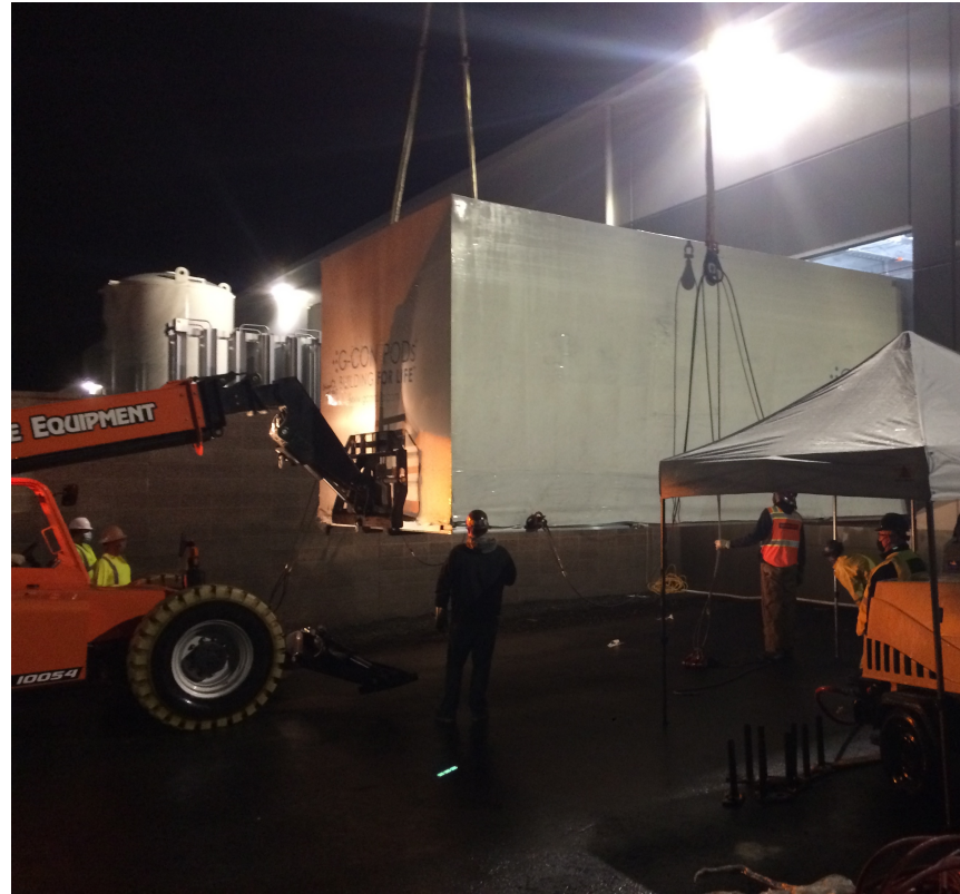
PODs moving into facility
