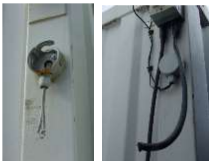
Damage to Wiska box and damage to electrics
