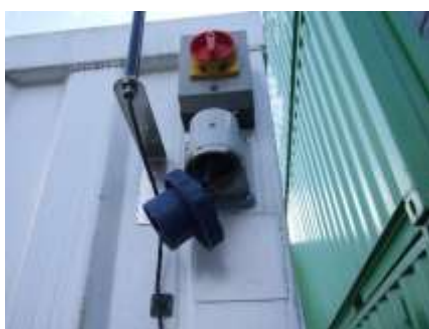
Damaged Commando Socket
