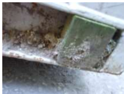
Concrete splashes on base of unit
