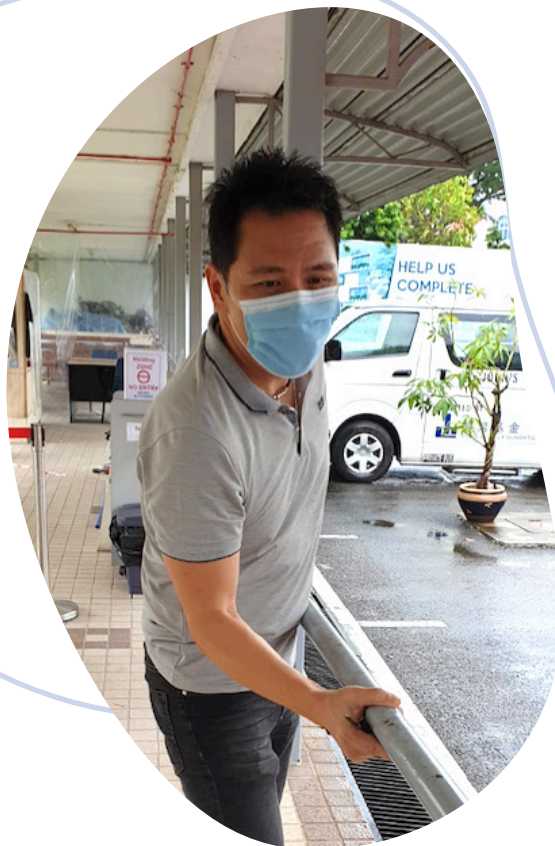
Andy putting up safe-distancing barriers to get the Home ready for Phase 2.
