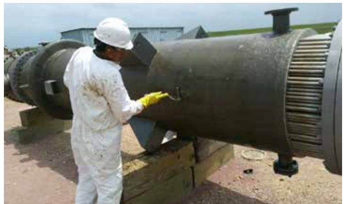
Our field technicians will complete a repair or new installation while adhering to customer specifications and safety guidelines.
