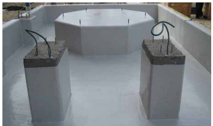
Concrete can be restored and/or protected from harsh chemicals resulting from leaks and spills.
