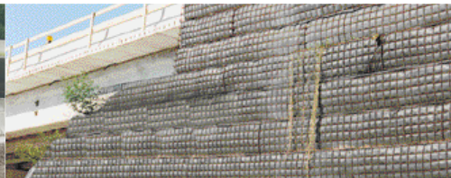
I-95, Florida – The Tensor Temporary Wall allowed the contractor to sequence construction to meet the bid budget and construction plan.
